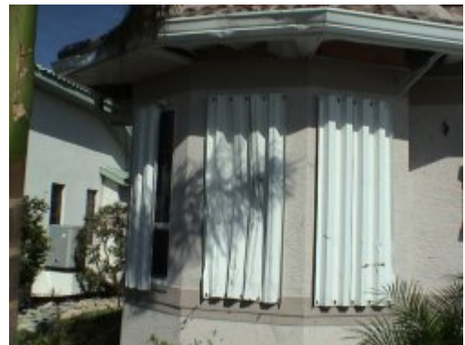
Tiles from surrounding roofs banded up these shutters
